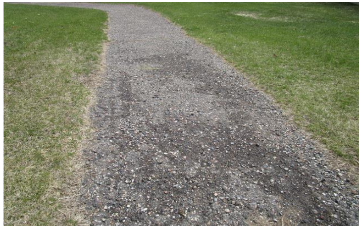
Failing pavement near south tennis courts
