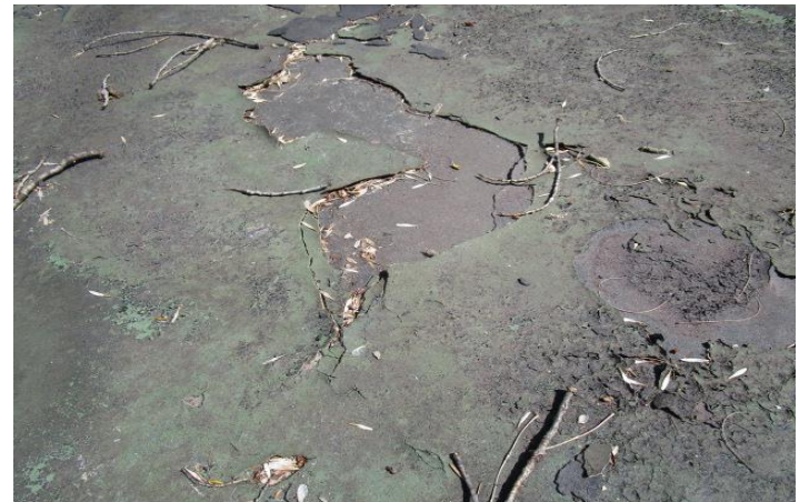
Failed color coat
