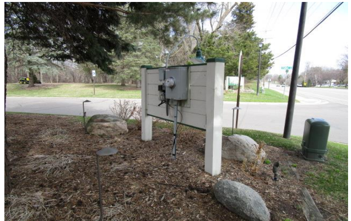
Recently added electrical equipment
