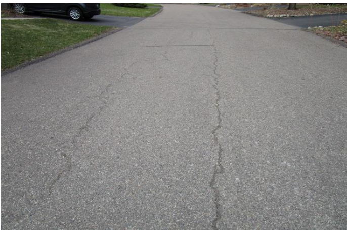
Longitudinal cracks at street
