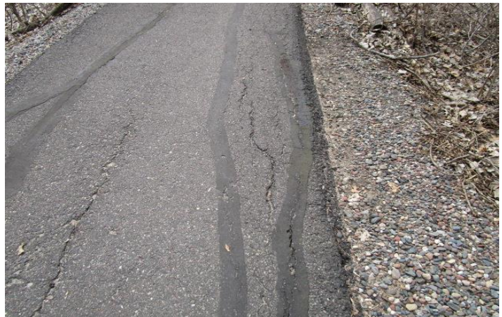
Repaired and unrepaired cracks
