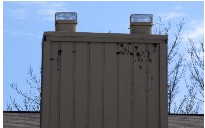
Siding deterioration at chimney chase
