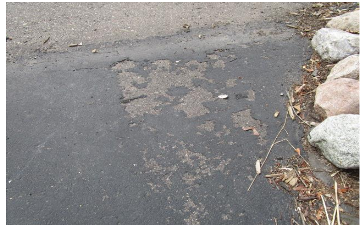
Isolated failing seal coat
