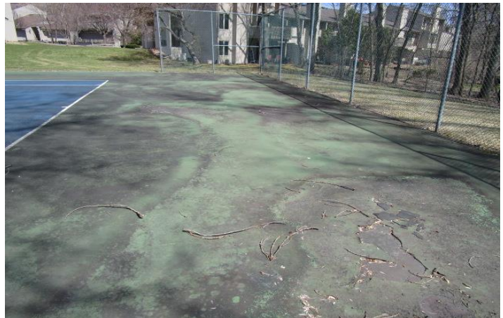
Discoloration of color coat
