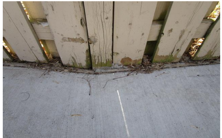
Wood rot at fence base
