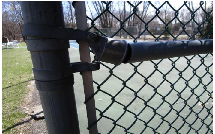
Loose rail connection
