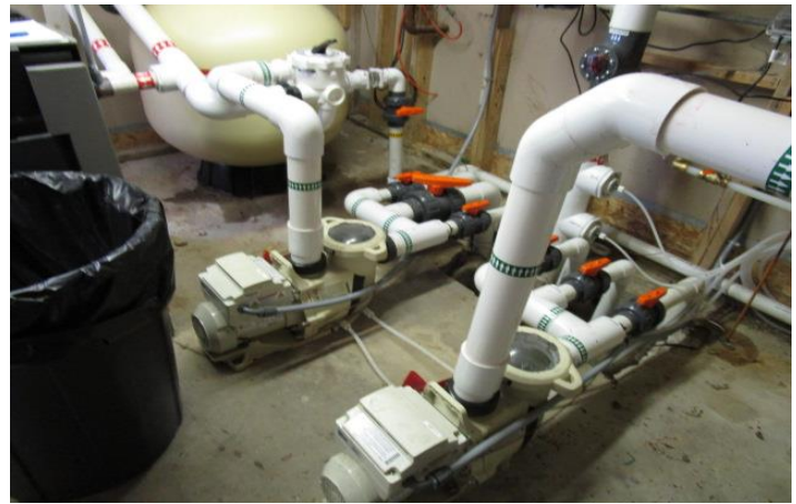
North pool pumps
