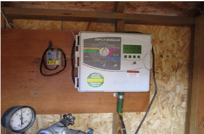
Irrigation system controller
