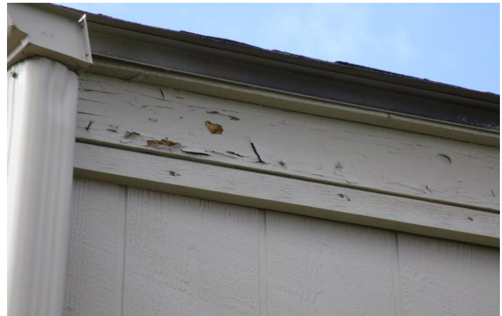
Poor paint finish at fascia
