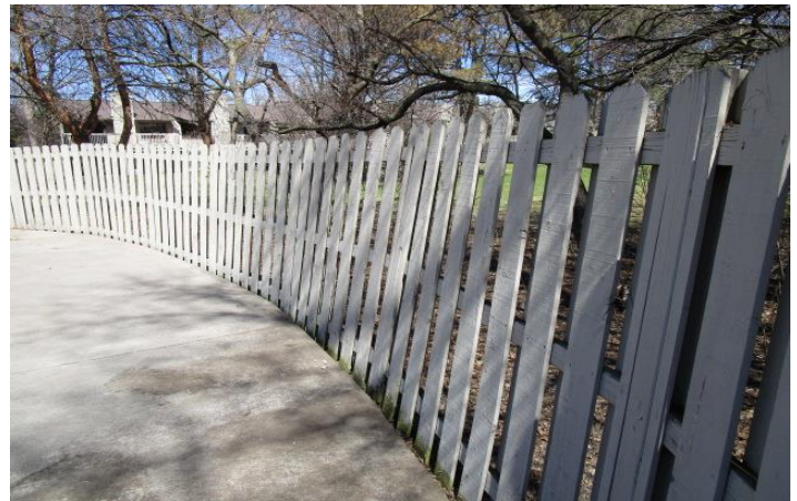
Leaning wood fence at south pool
