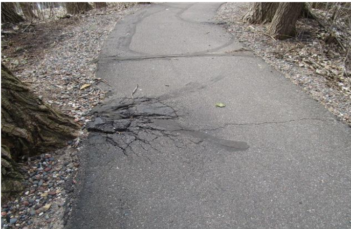
Trip hazard at walking path
