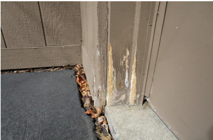
Chipped paint finishes at garage trim
