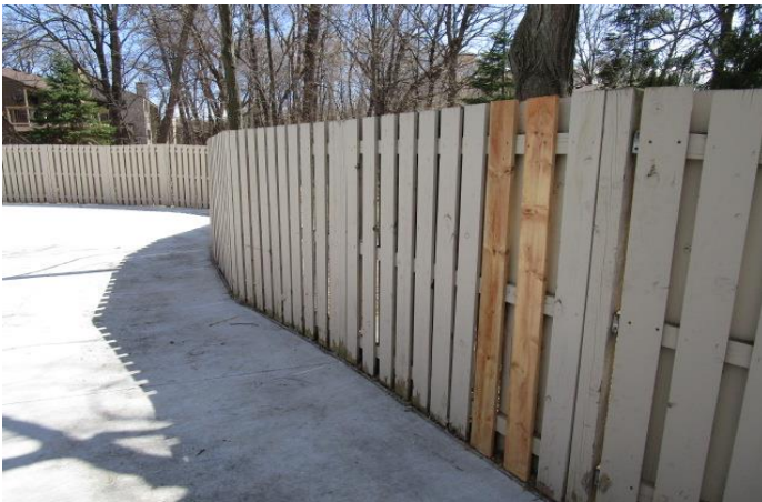
Previous wood board replacements
