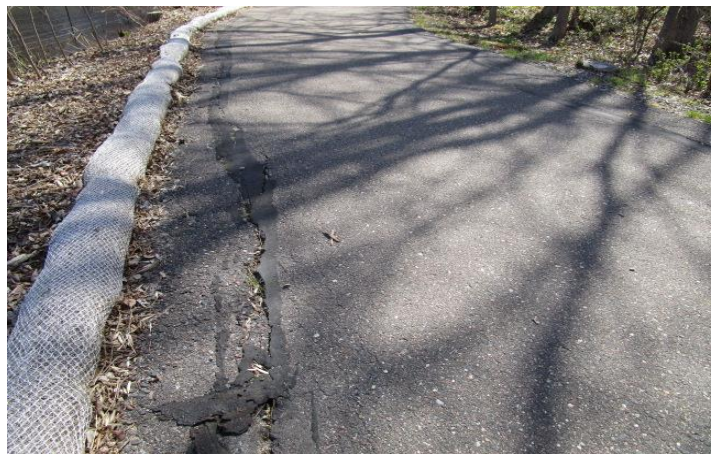
Longitudinal cracks at street
