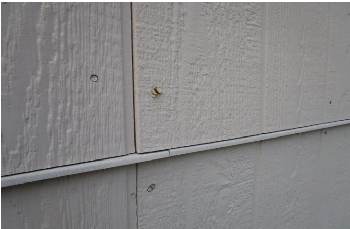
Rust at fastener
