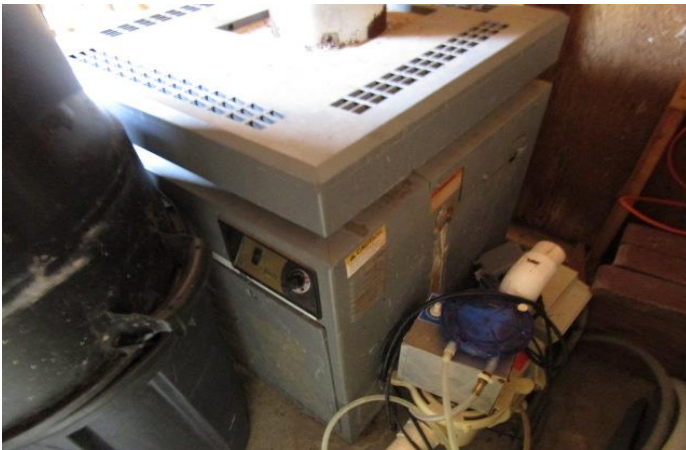
South pool heater
