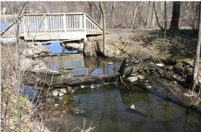
Weir in poor condition
