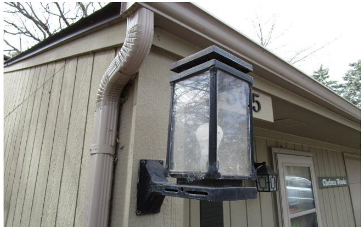
Aluminum gutter and downspout
