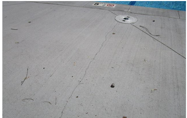
Hairline crack at north pool deck
