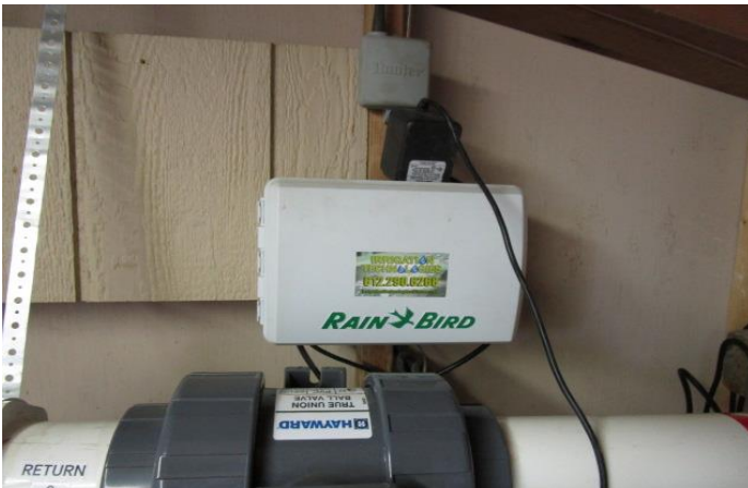
Irrigation system controller
