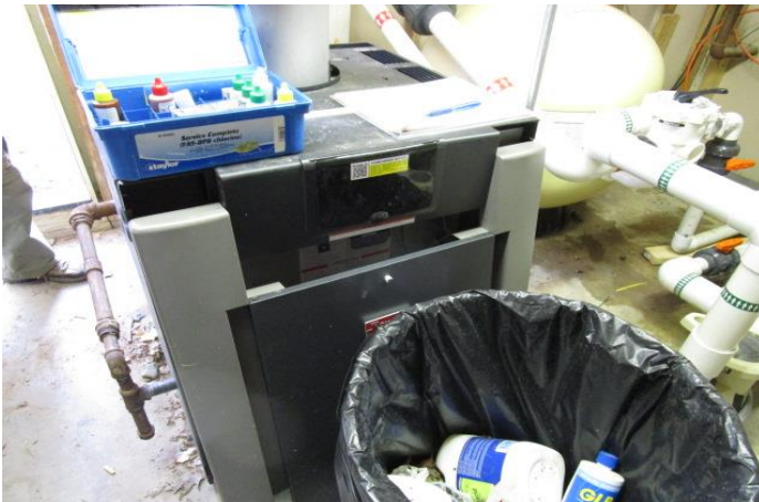
North pool heater
