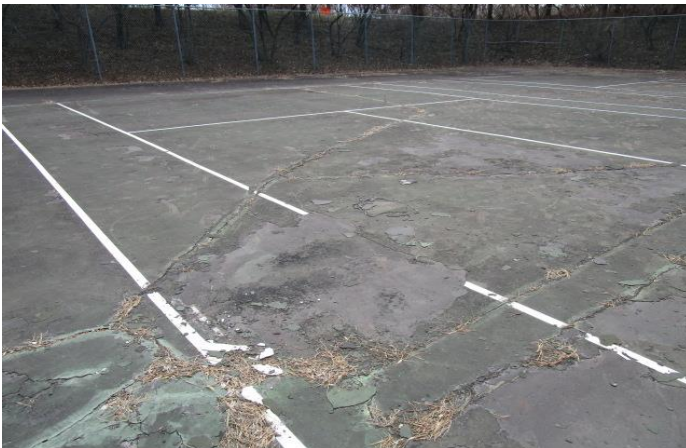
Failed color coat and cracks
