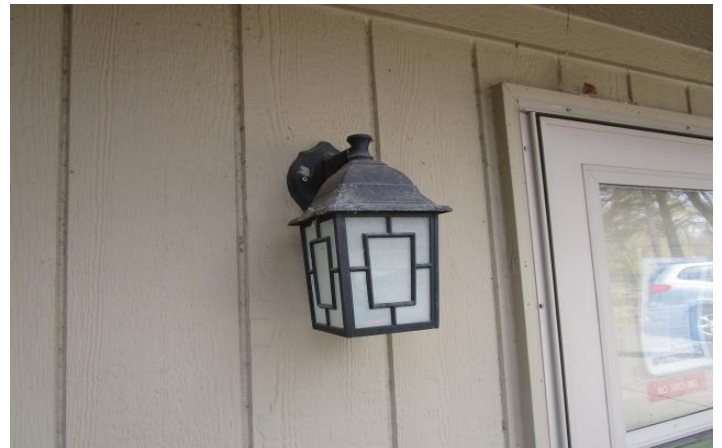
Light fixture at office
