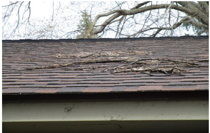
Debris on roof
