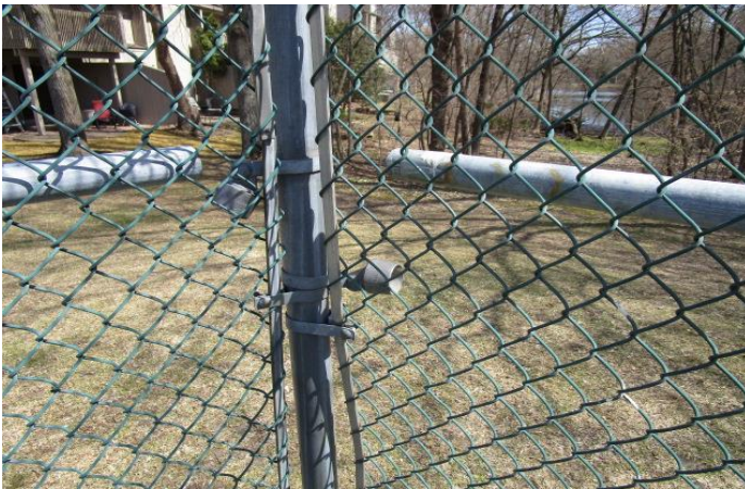
Loose rail connections
